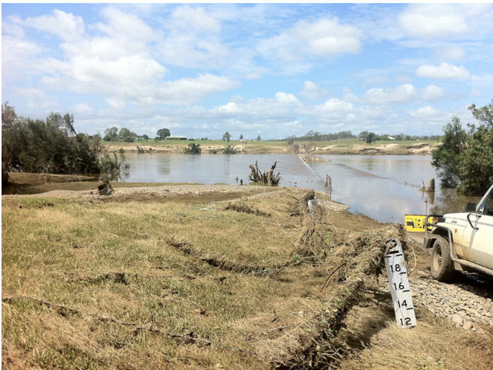
Rogans Bridge, Clarence River (post-flood), 11.20 am, 2 February 2013
